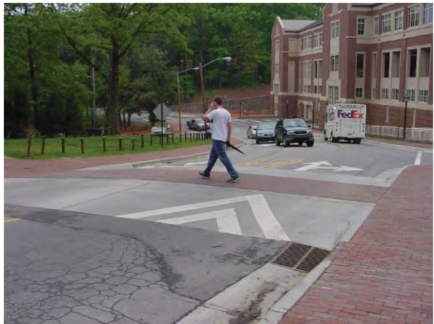
Raised crosswalk: University of North Carolina Campus, Chapel Hill, NC (Credit: Ryan Snyder)
